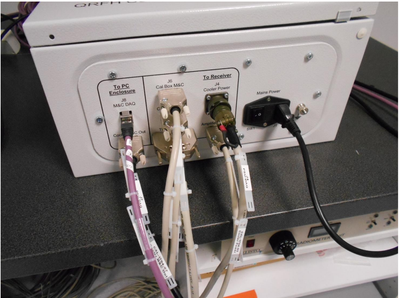
Figure 6-1: DAQ-PSU Enclosure - Cables routing space
